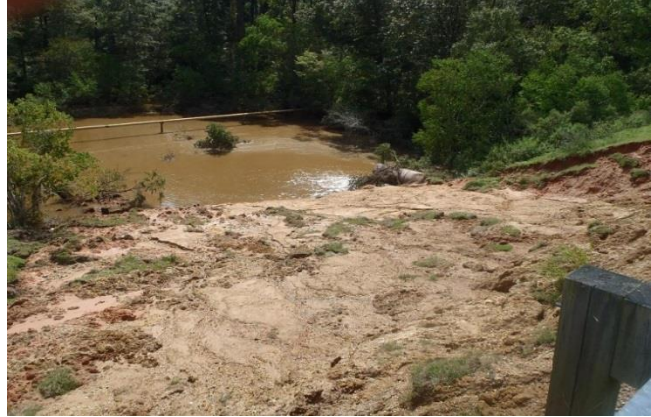
Landslide on the Percy Quin State Park dam caused by Hurricane Isaac
